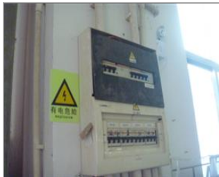
Photo of non-conformity NC No cover.JPG
