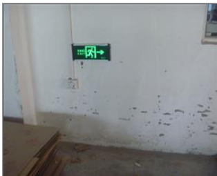
Photo of fire safety equipment evacuation sign.JPG
