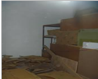
Photo of non-conformity NC Materials stored against the wall.JPG
