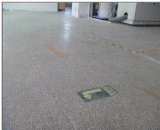
Photo of fire safety equipment evacuation ailes.JPG
