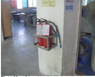
Photo of fire safety equipment fire extinguishers.JPG
