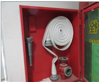
Photo of fire safety equipment Hydrant inside view.JPG
