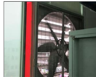
Photo of the inside of the main production hall Ventilation fan in production workshop.JPG
