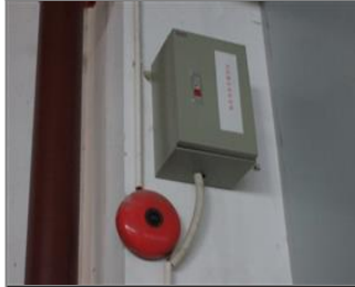
Photo of fire safety equipment Back up power to fire alarm.JPG
