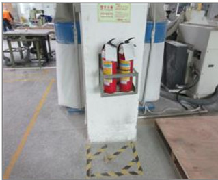
Photo of fire safety equipment Fire extinguishers.JPG
