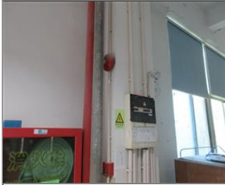
Photo of fire safety equipment Fire alarm.JPG
