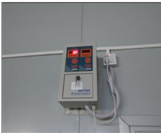
Photo of fire safety equipment Gas monitoring machine.JPG
