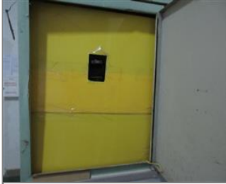
Photo of fire safety equipment inside view of electricity distribution box.JPG
