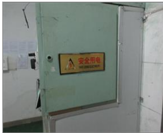
Photo of fire safety equipment Electricity distribution box.JPG
