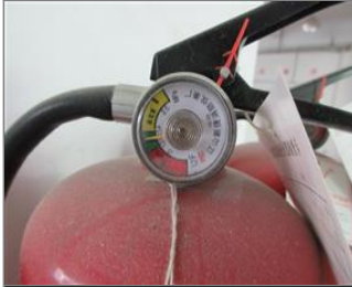
Photo of fire safety equipment Extinguisher with normal pressure.JPG
