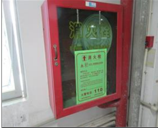
Photo of fire safety equipment Hydrant.JPG
